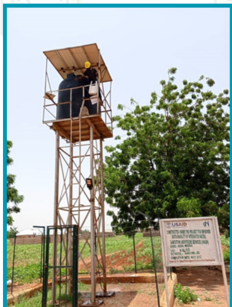
Constructed Solar-Powered Borehole at Dangoma JSS Kalgo LGA, Kebbi State During the I-WASH Project, 19th August 2024.
